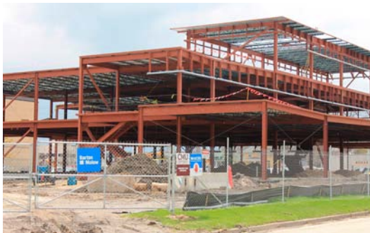
The Central Michigan University College of Medicine East Campus is located at the northeast portion of Covenant HealthCare's main campus in the City of Saginaw.
