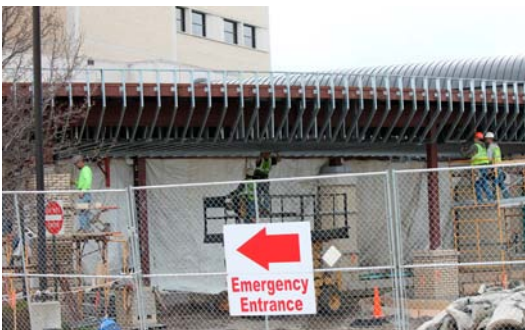
The Covenant Healthcare Emergency Care Center is located at 900 Cooper Ave. in the City of Saginaw.
